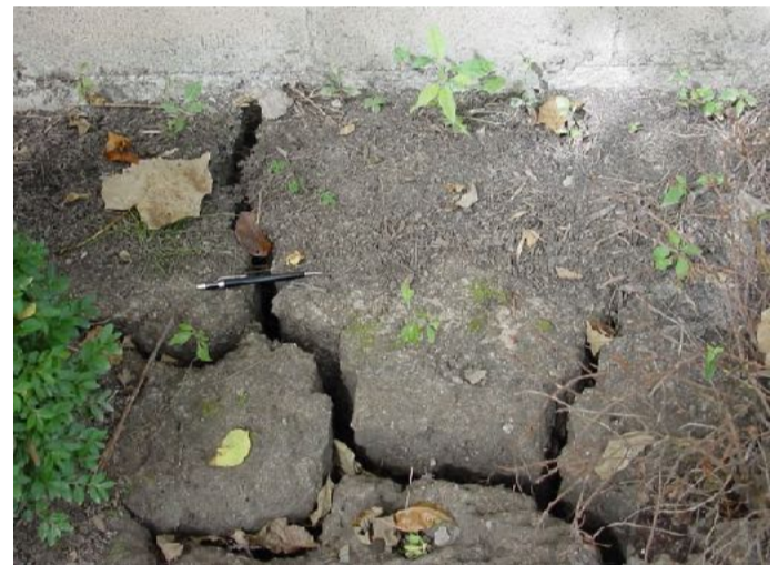
Fig 4 - Visual Appearance of Expansive Soils When Dry
